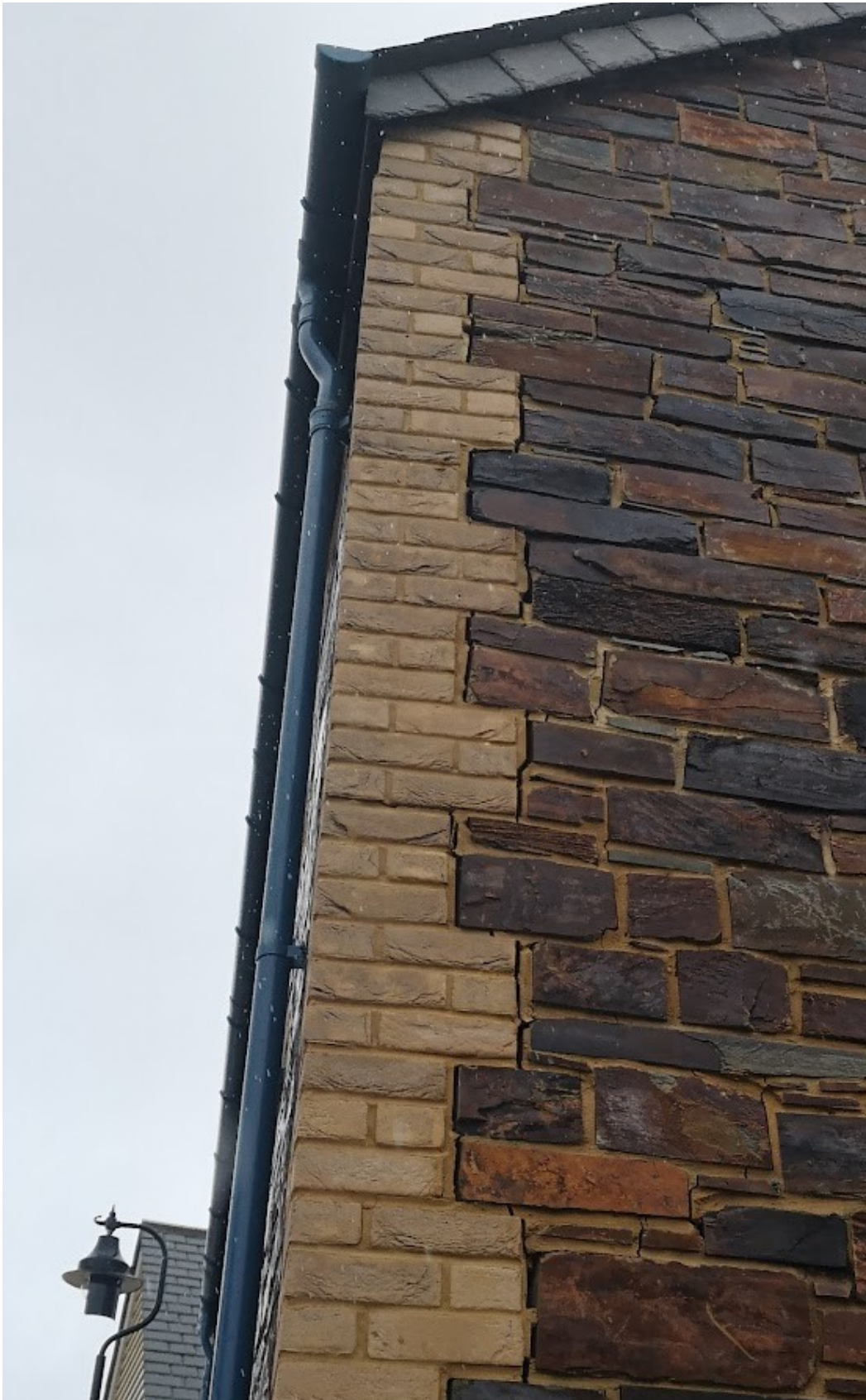
Example of stone and brick functioning adequately but serious mortar cracking between them suggests underlying movement or issues with the mortar mix. These cracks will likely lead to further damage over time, including to the stone units. Note the very fine sandy mortar that has been used.
