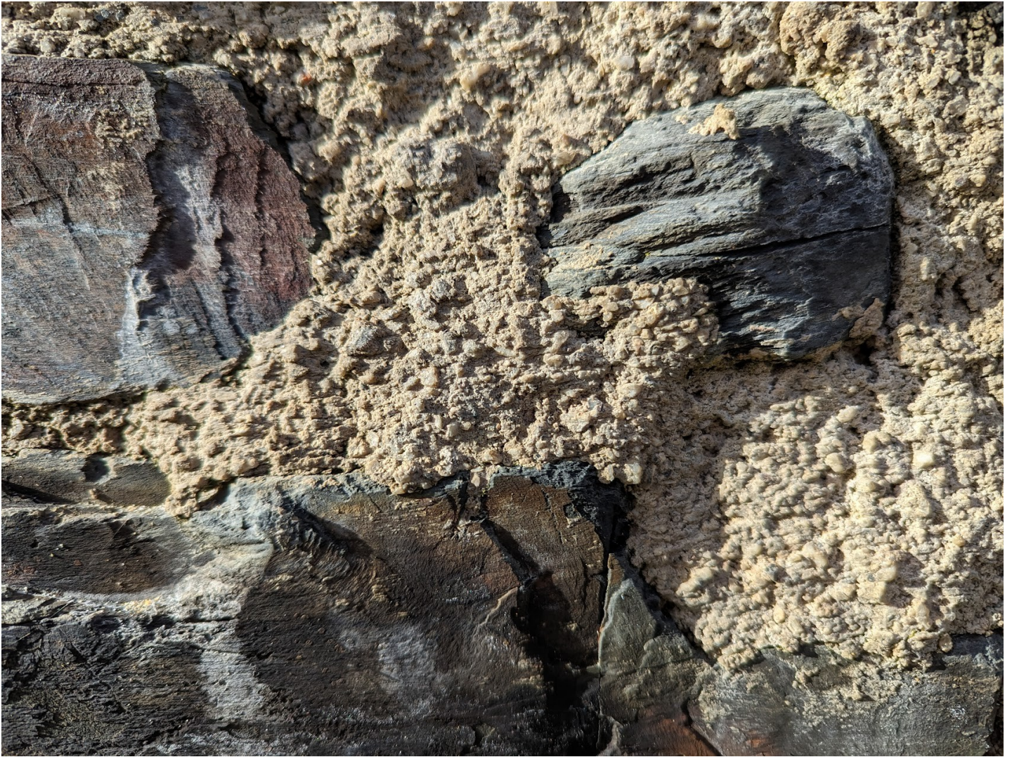
Example photo showing a very durable lime mortar with well graded, coarse aggregate size.
